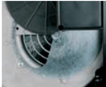
Air damper partially open
